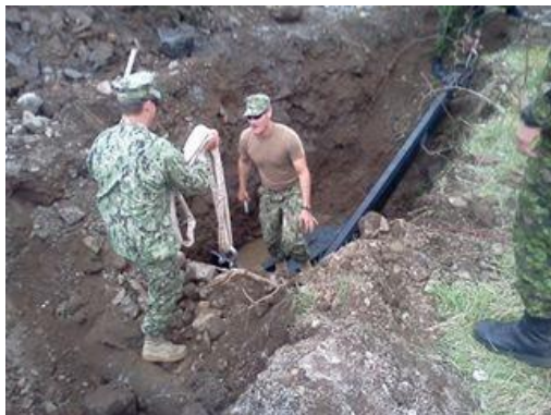
MUDSU2 workers installing 6,000 lb anchors to aid in righting Cape Ann III .
