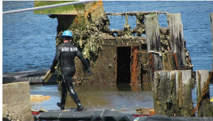
MUDSU2 worker scrambling to check plugs. The pumps had to drain the water faster than it was coming in, the plugs had to hold, and Cape Ann III had to be positive buoyant before slack tide was over. Oh ya, one plug failed (~6'x6') - they replaced it with just minutes to spare, and the ship became positive buoyant.
